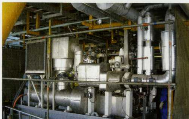
Leistriz high-pressure multiphase with heat tracing and insulation on a wellhead platform in Bobai Bay
